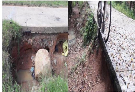
Fig. 5. Disintegration of Sub Base
