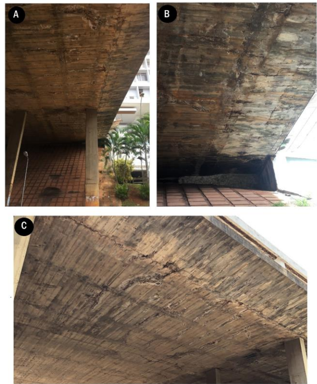
Fig. 2. Lateral edge with the presence of efflorescence, exposed reinforcement, dirt, cracks and cracks
