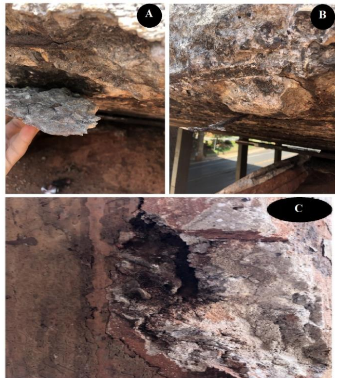
Fig. 6. A) Cracking of the concrete in the tray; B) Fragility in concrete, peeling point; C) Abutment of the concrete in the pillar
