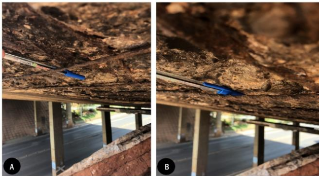
Fig. 5. Exposure and corrosion of reinforcement.
