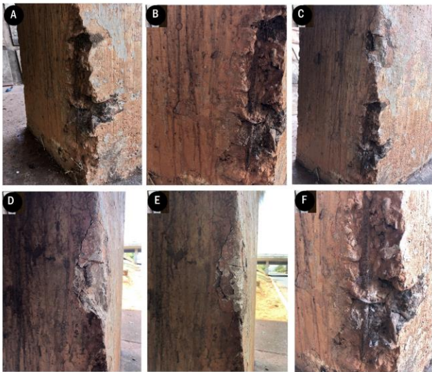
Fig. 1. Reinforcement exposed in different pillars of the bridge
